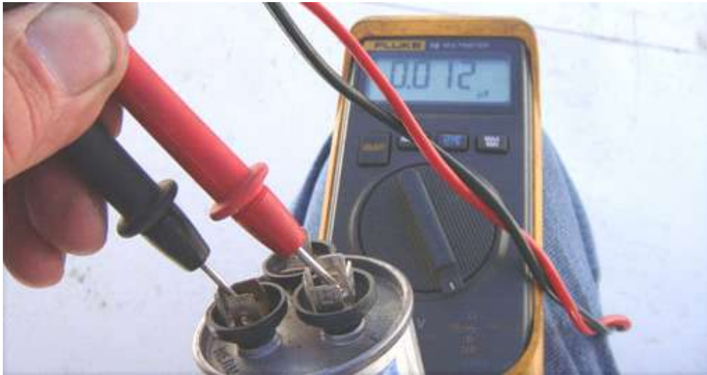
Figure 6.5 Checking 50 \mu\text{F} capacitor but only measuring 0.012 \mu\text{F} indicating failure
