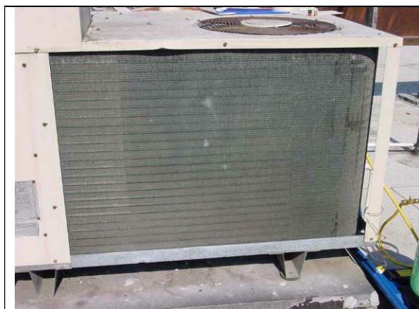
Figure 2.1 Dirty Condenser Coil
